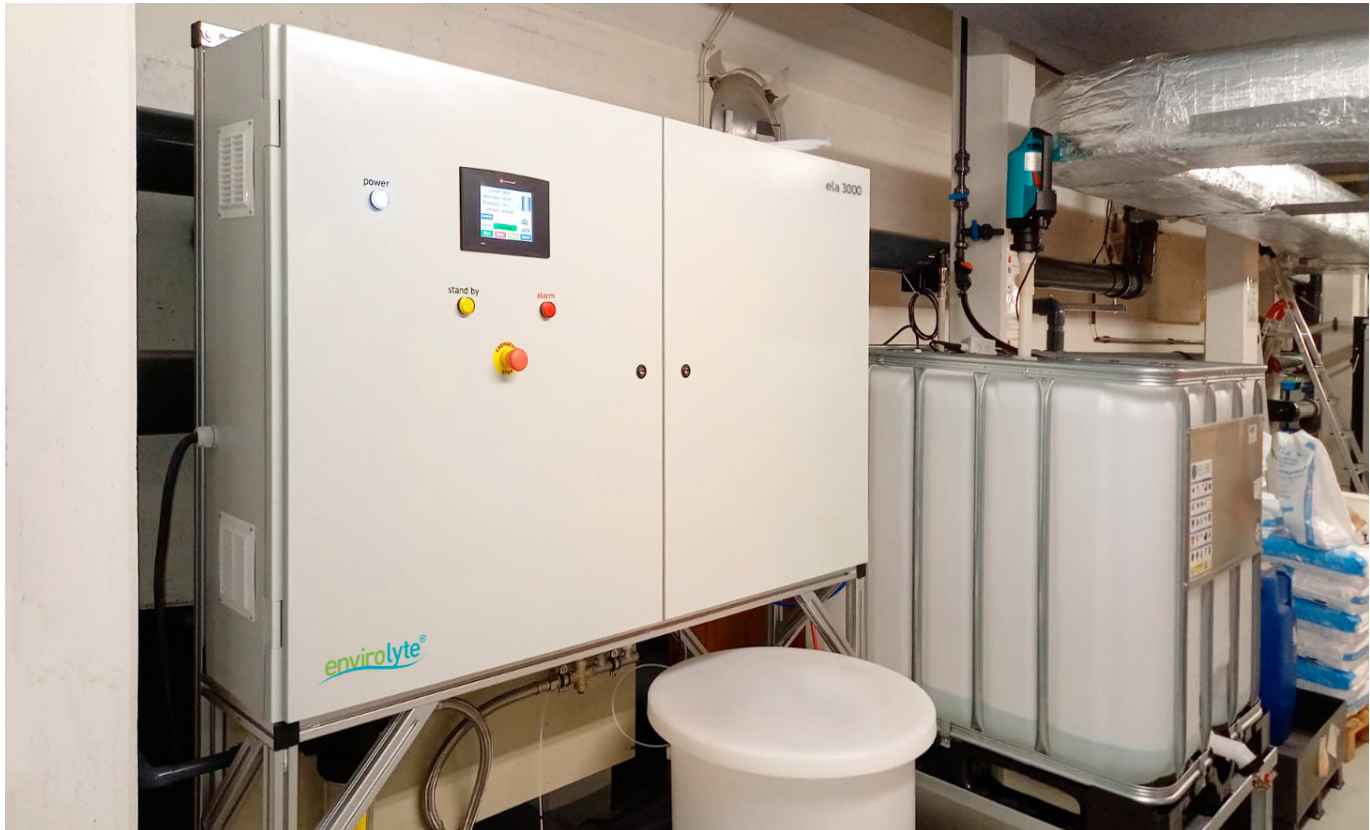
On site installations of ela3000
