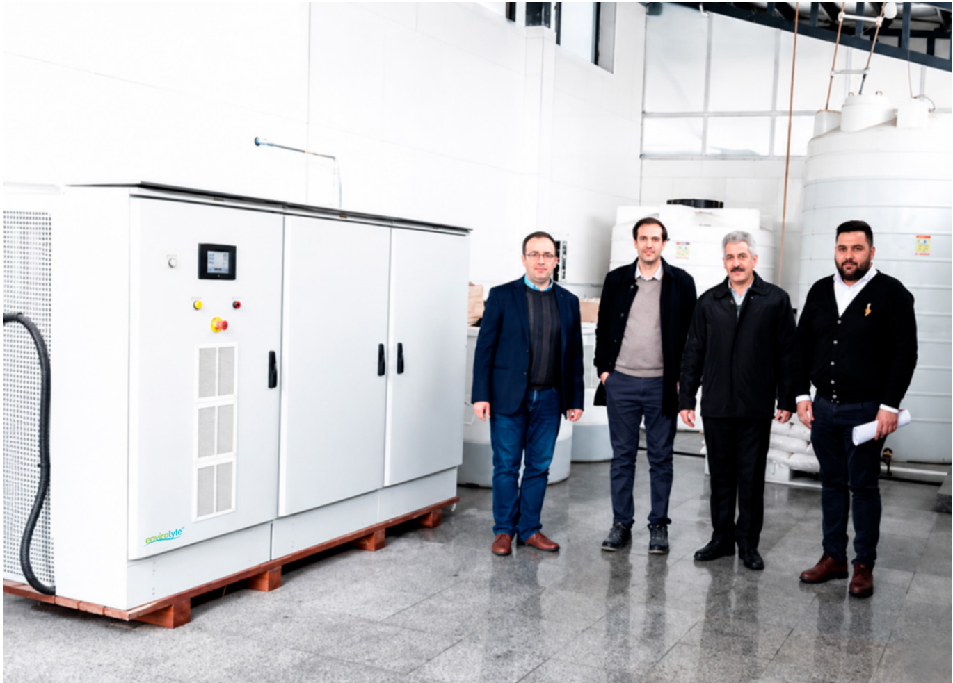
On site installations of ela50000ANW
