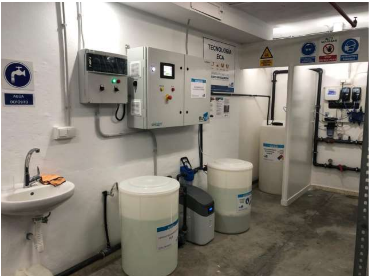
Envirolyte ELA-200ANW with anolyte and brine tanks and water softener.
