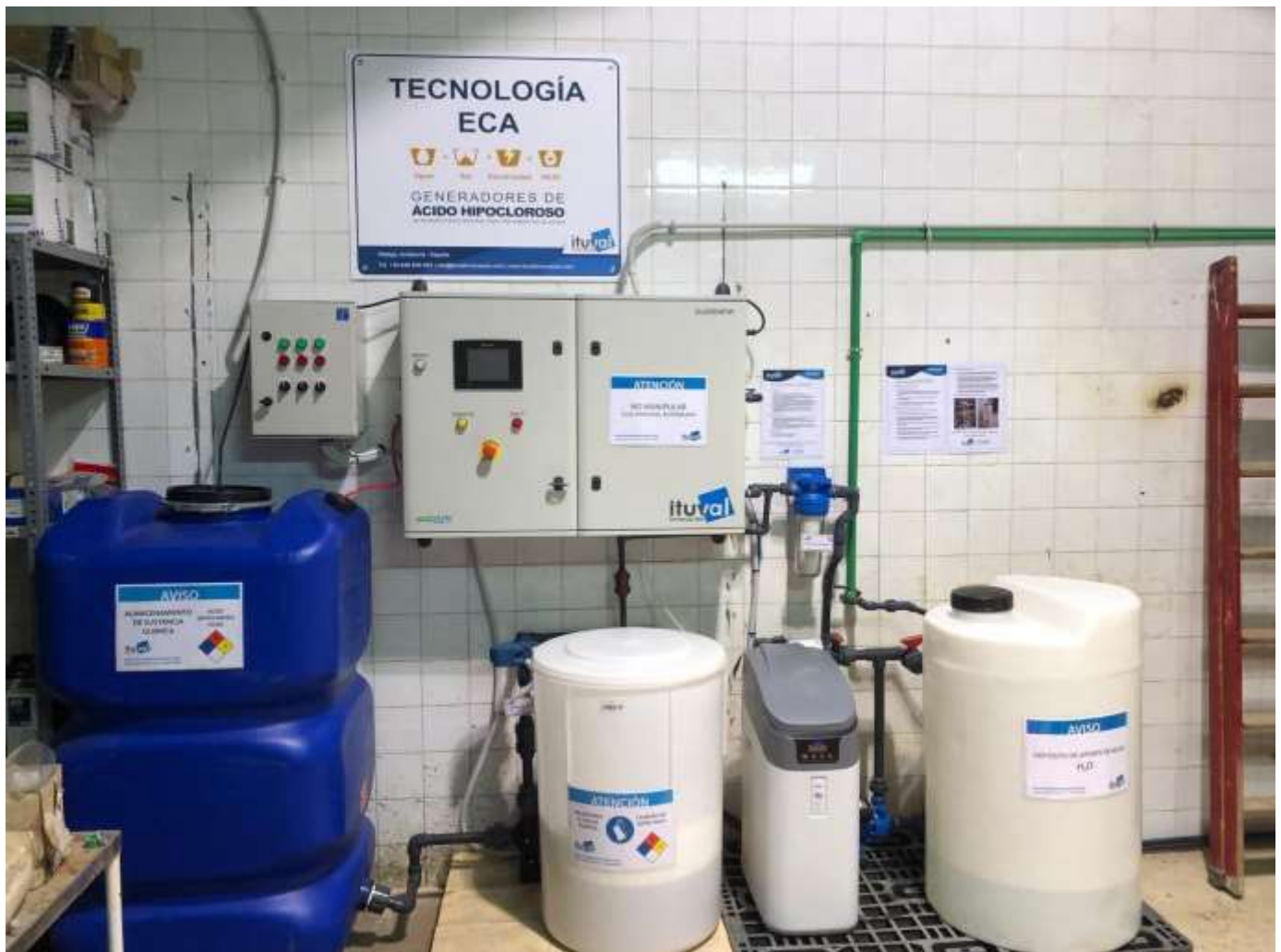
Envirolite ELA - 900ANW with brine tank, storage tank and water softener
