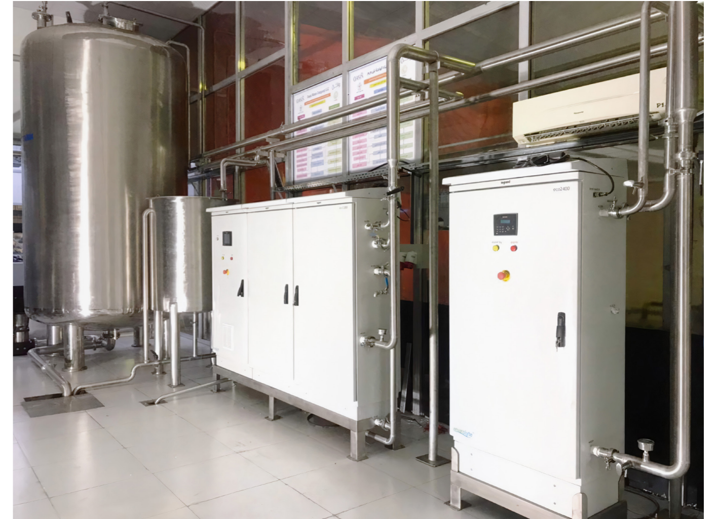
Envirolyte ECO alkaline ionized water generators in Oman
