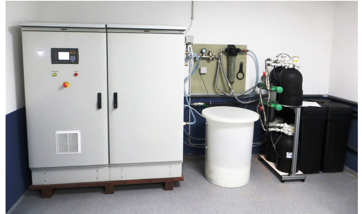
Envirolyte ela18000 generator in Germany with installation accessories
