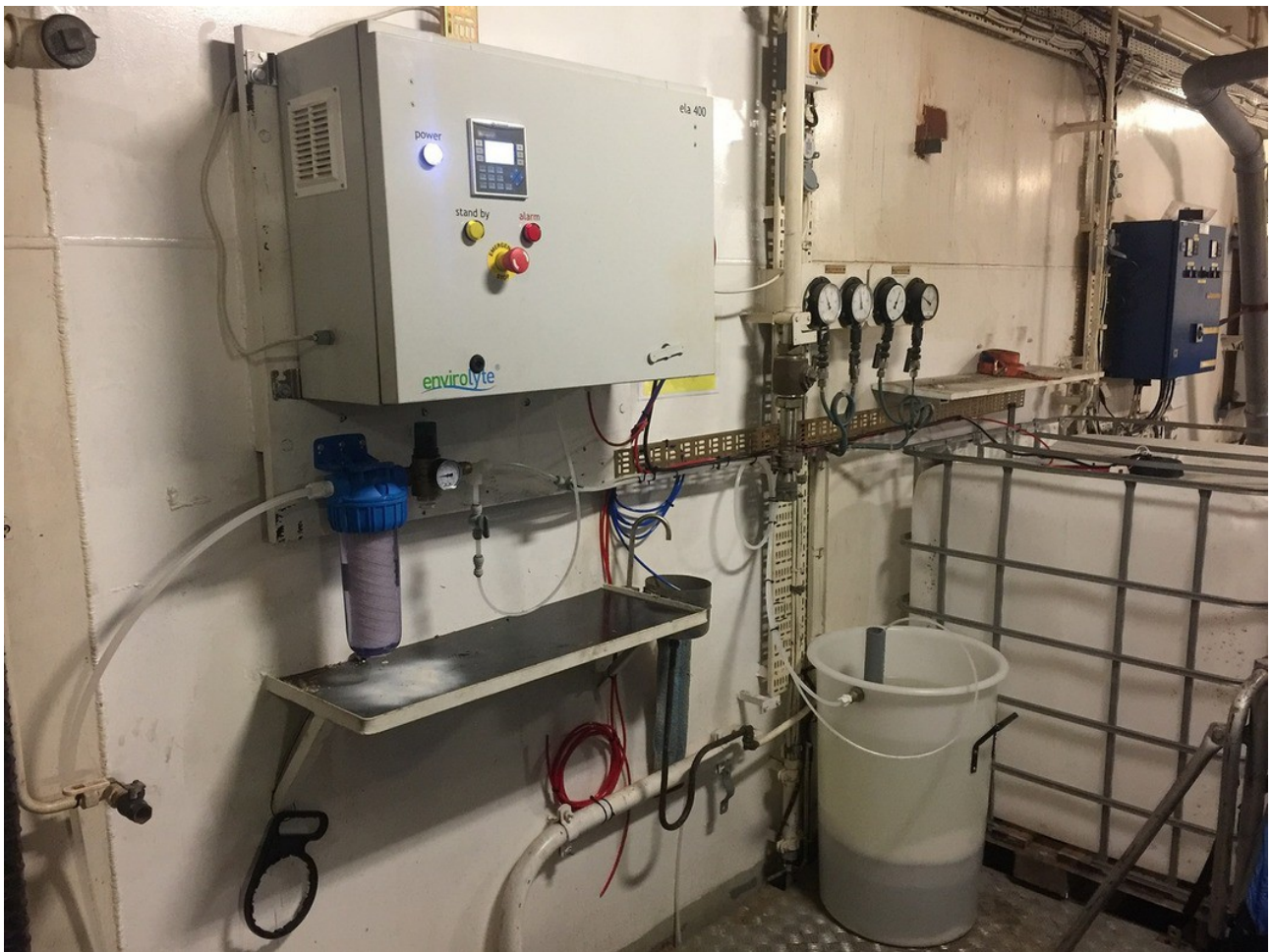
General view of ELA-400 with anolyte storage tank
