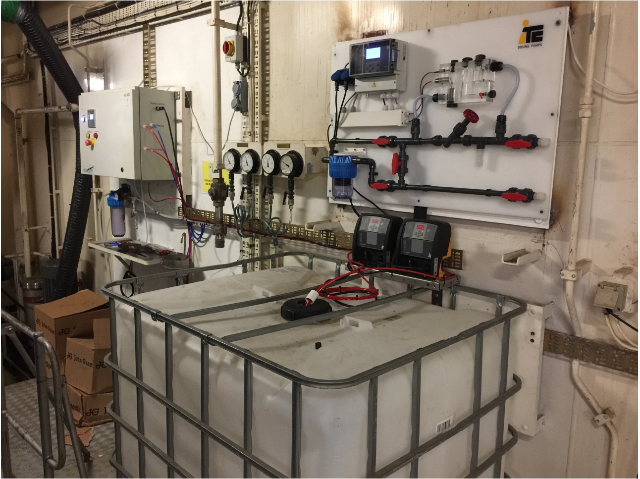
Enviolyte ELA-400 anolyte generator with anolyte storage tank
