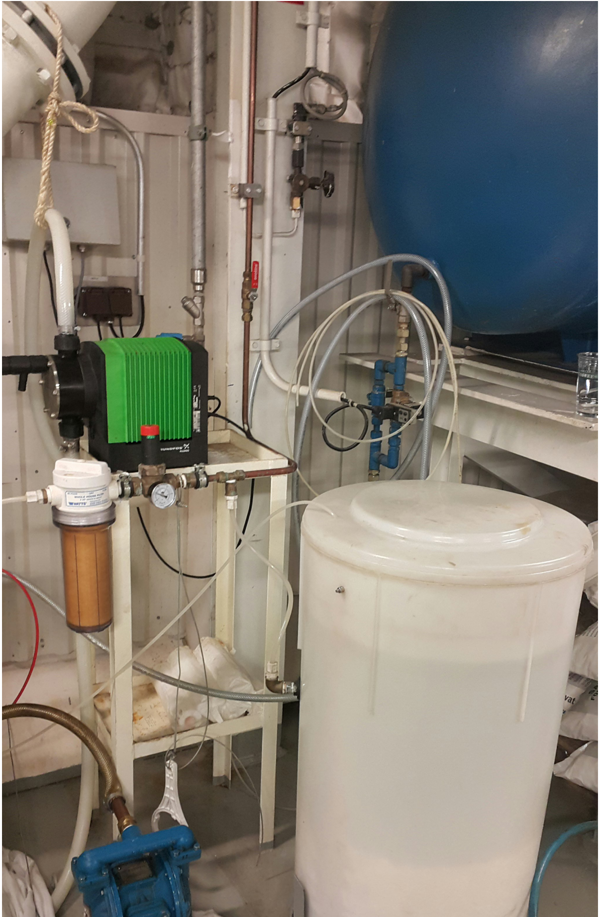
Analyte dosing pump with brine tank and water filter
