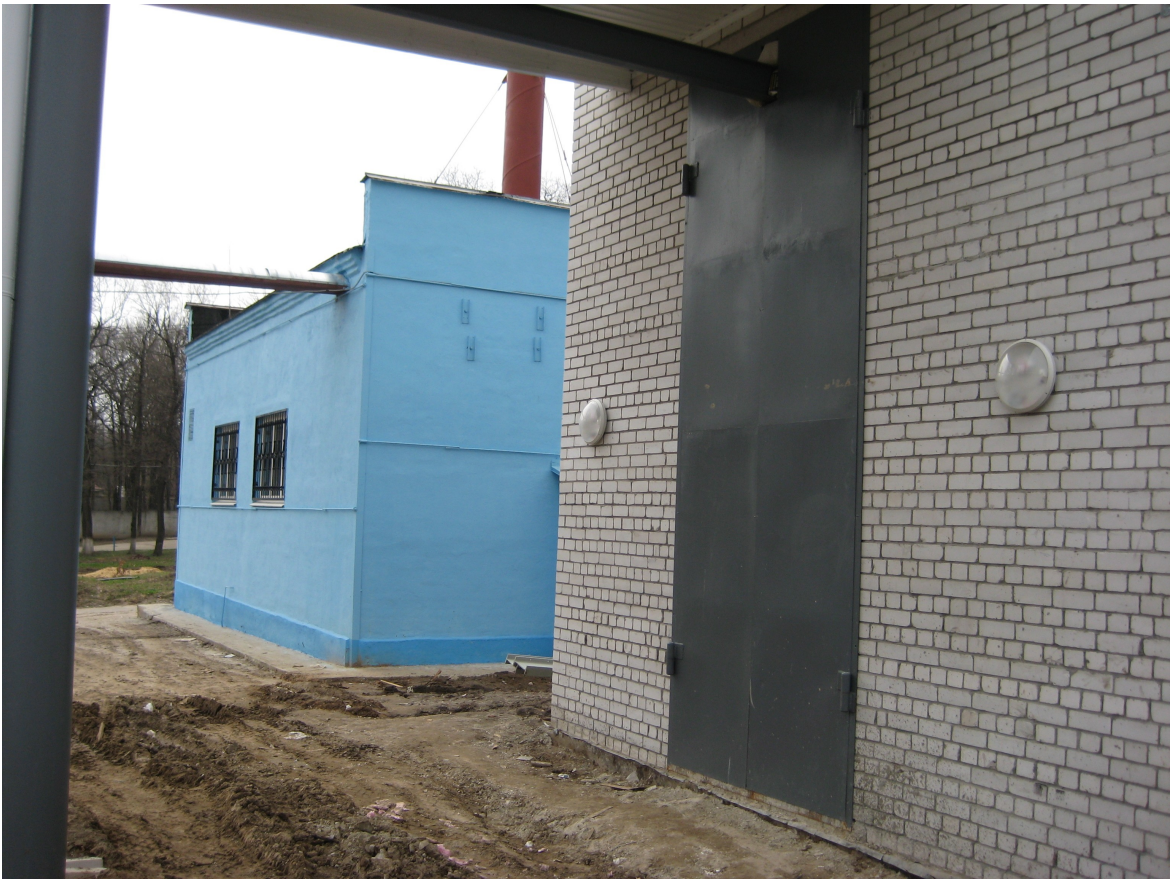
Booster station/installation site
