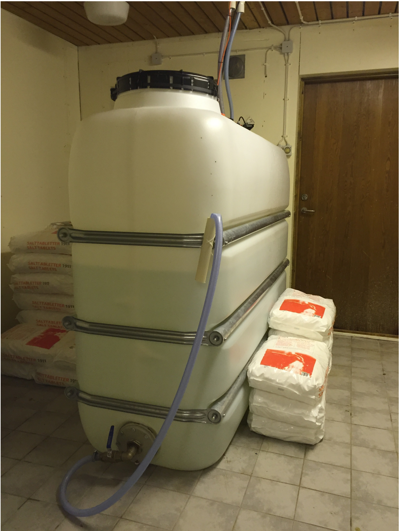
Anolyte storage tank
