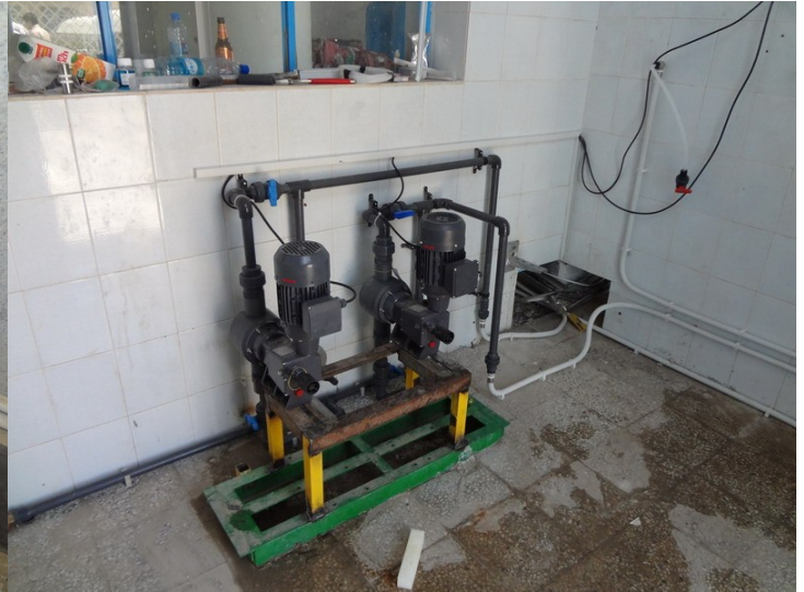
Anolyte injection pumps
