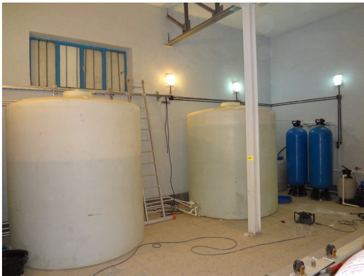
Anolyte tank and water softeners
