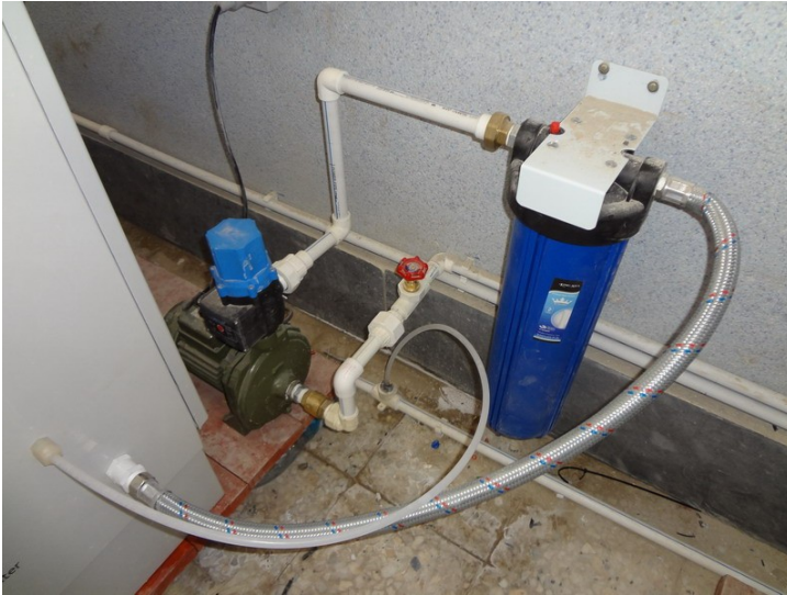
Source water pre filtration
