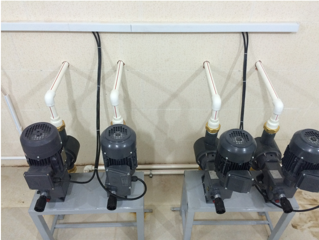
Anolyte injection pumps. Dosing 1ppm at the injection point.
