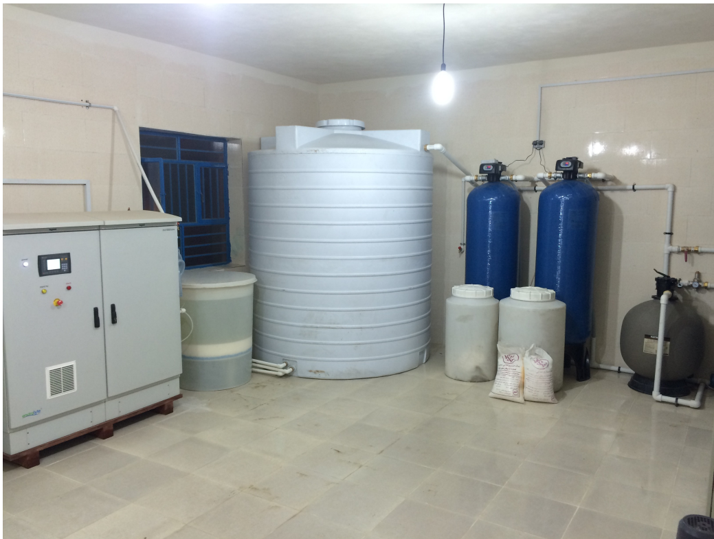
ELA-18 000ANW with brine and anolyte storage tanks
