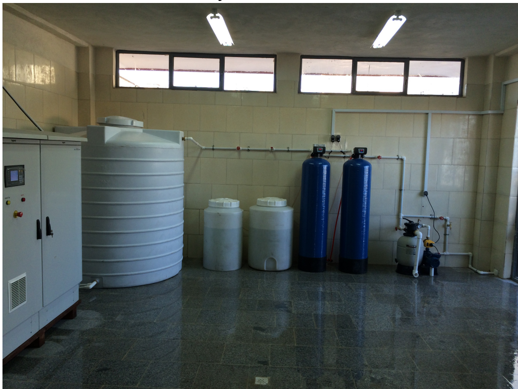
ELA-10 000ANW with brine and anolyte storage tanks, water softeners and dosing pump. Dosing 2 ppm at the injection point.
