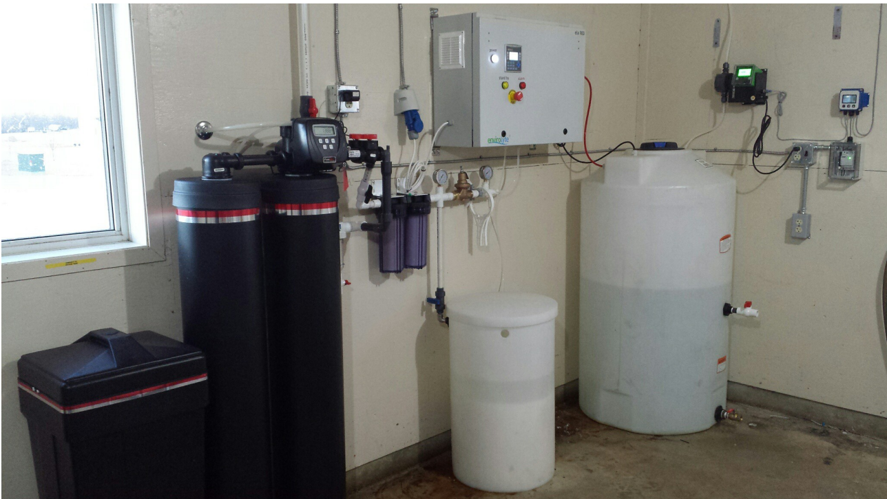
Enviolyte ELA-900 generator with water softener, brine and anolyte storage tanks, dosing pump and flow meter
