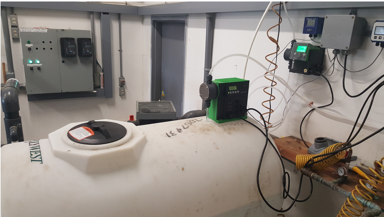
Analyte tank with dosing pump
