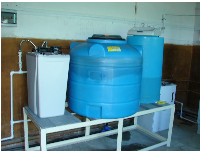
Water softener and brine tanks
