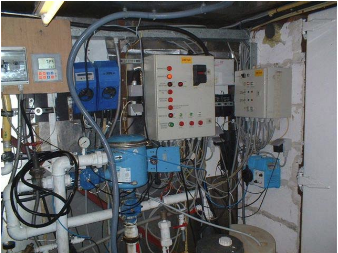
The engine/installation room with different control systems
